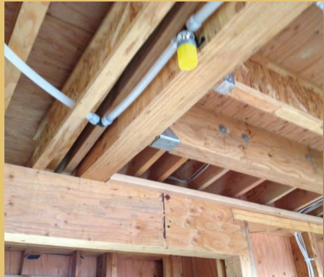
FIGURE 8 Right: A residential sprinkler system showing pipe routing and support.
